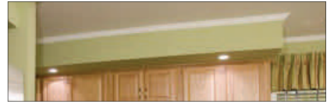
LIGHTED SOFFIT (MODS ONLY) & CAN LIGHTS
